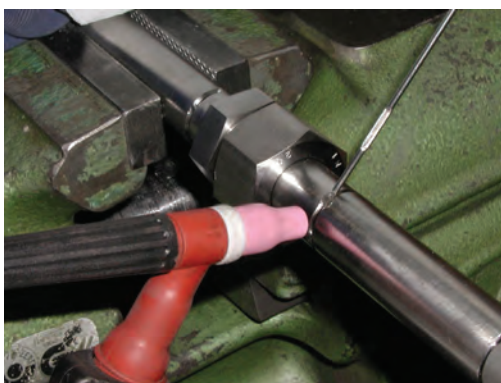
3. Tack-welding when bolted together. Clamping nut slightly tightened. Pay attention to the negative pole.
